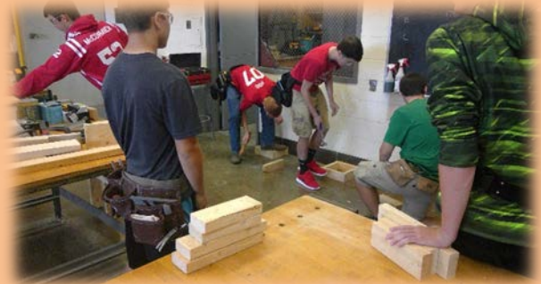
Students in Mr. Burr's Building Trades classes practice their framing and hand tool skills.
